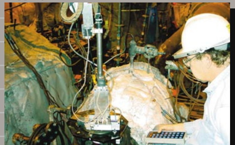
On-site and in-place orbital TIG welding of worn and cracked Governor valve seats are repaired using custom-designed equipment and remote control operation.
