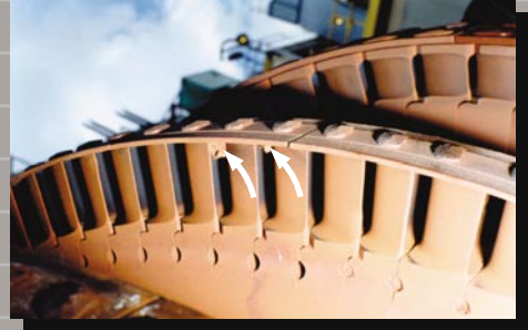
Foreign objects that can impede steam flow are identified and their impact on efficiency quantified during steampath inspections.
