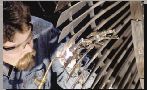
Erosion shield installations and replacements on LP rotors can be conducted on-site or in one of MD&A's repair facilities.
