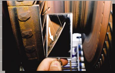
Structural audits identify erosion under bucket covers and shroud bands that can affect the structural integrity of a stage.
