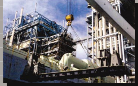
Set up of portable lathes can be completed within a twelve hour shift and require no drilling or anchors that could damage the turbine deck.
